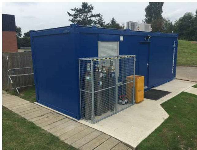
Figure 1. Installation at Affinity Water's treatment works.
