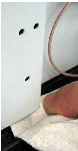
Fig. 40: Drying the leak sensor
