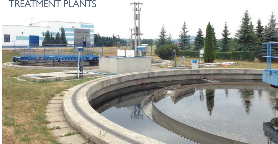
MUNICIPAL WASTEWATER TREATMENT PLANTS
