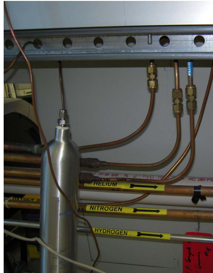
Infrastructure Plumbing Not so easy access
